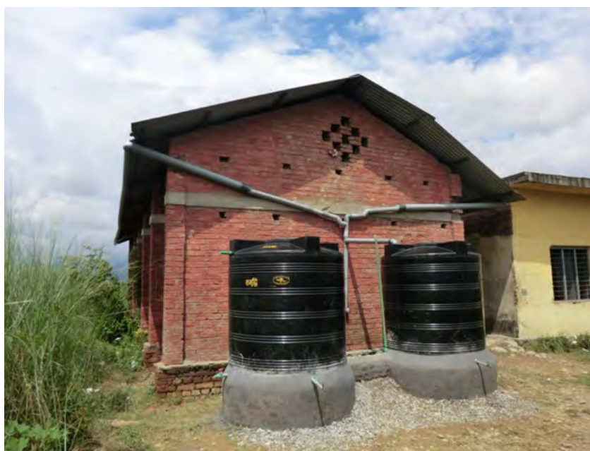
Photo. 6.1 Water Tanks and the Piping Systems for Rainwater Harvesting
