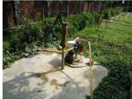
Photo 5.6 Well with motor pump (School in Khokharpurwa)
