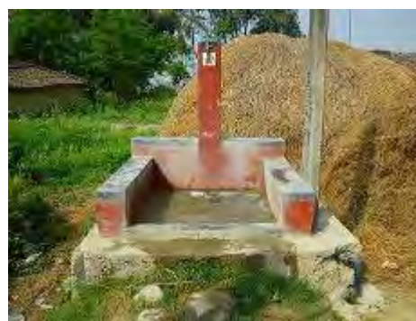
Photo 5.2 Waterworks Facility (Goini) Joint Water Place Connected from the Water Tower of Photo 5.1 Usage Fee; 70 rupees per month Supplying Time: about 2 hours per day
